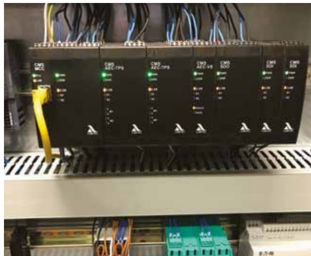
CMS modules installed in the control cabinet.
