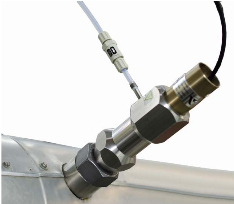
Fig. 5-3 Testing device plugged into flue gas channel
