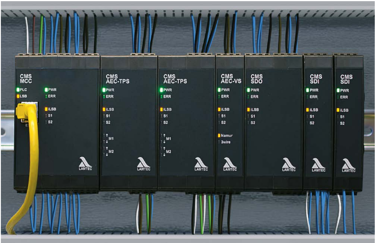
CMS in operation
